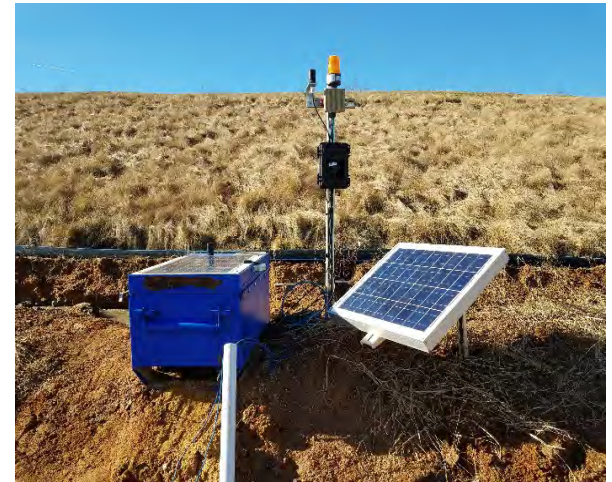
Solar Powered “Real-time” Porewater Pressure Monitoring
